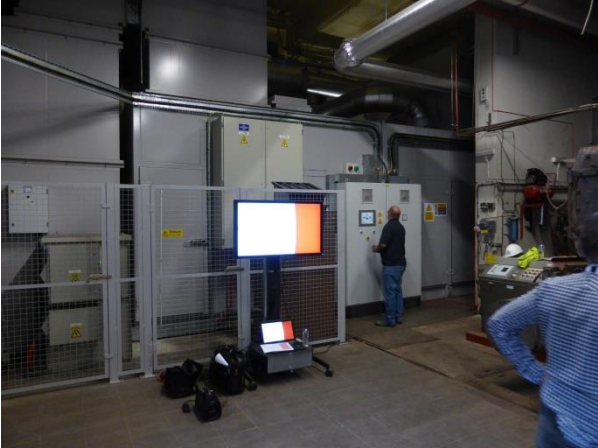
CHP Plant and control
