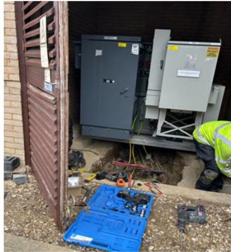
New HV Transformer
