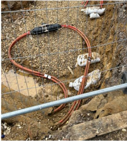
HV Cable Joint
